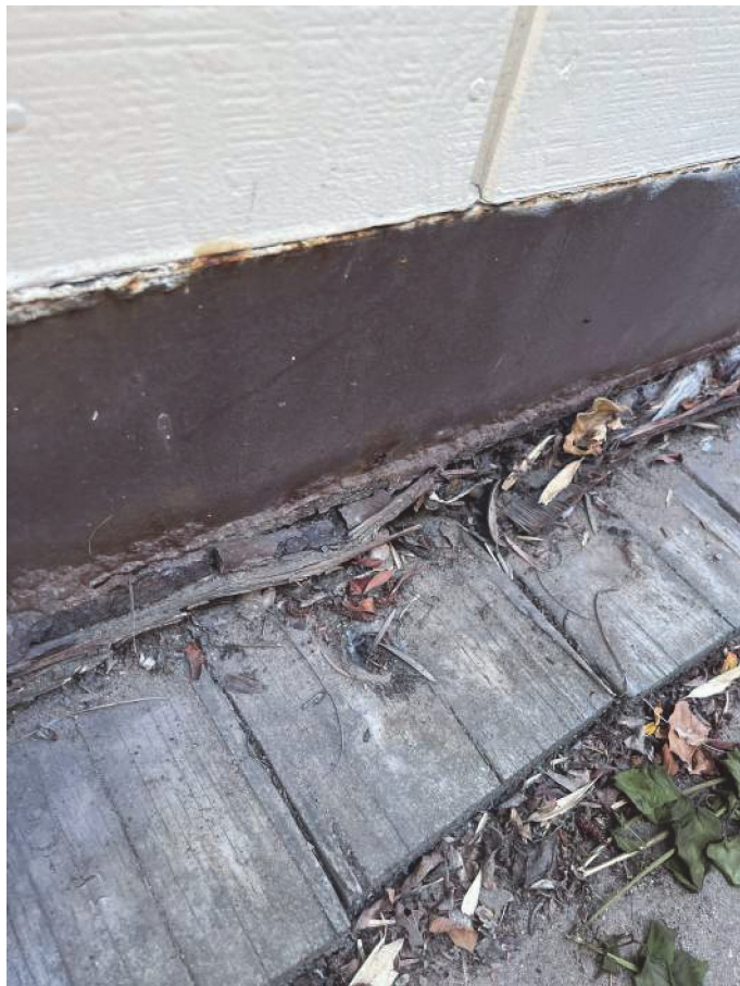
Damage to Plywood Skirting/Wood Sill
