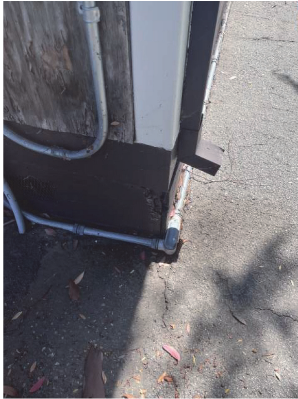
Slight Deterioration to Cripple Wall Sheathing
