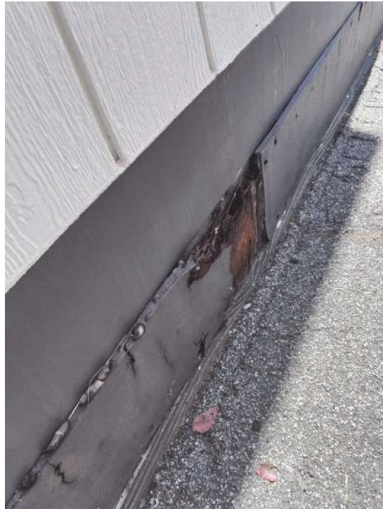
Damage to Plywood Skirting
