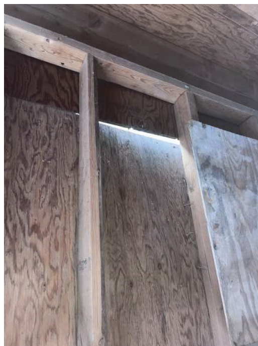
Building 37 - Damage to Exterior Wall Sheathing
