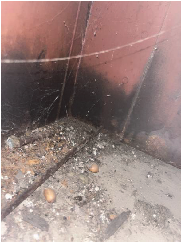
Slight Deterioration of Floor System on Footing
