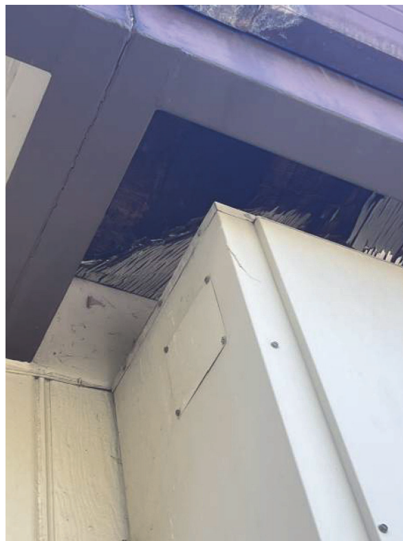
Damage to Plywood Roof Sheathing
