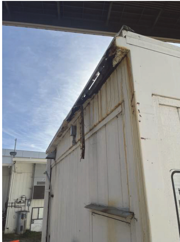
Significant Damage to Gutter
