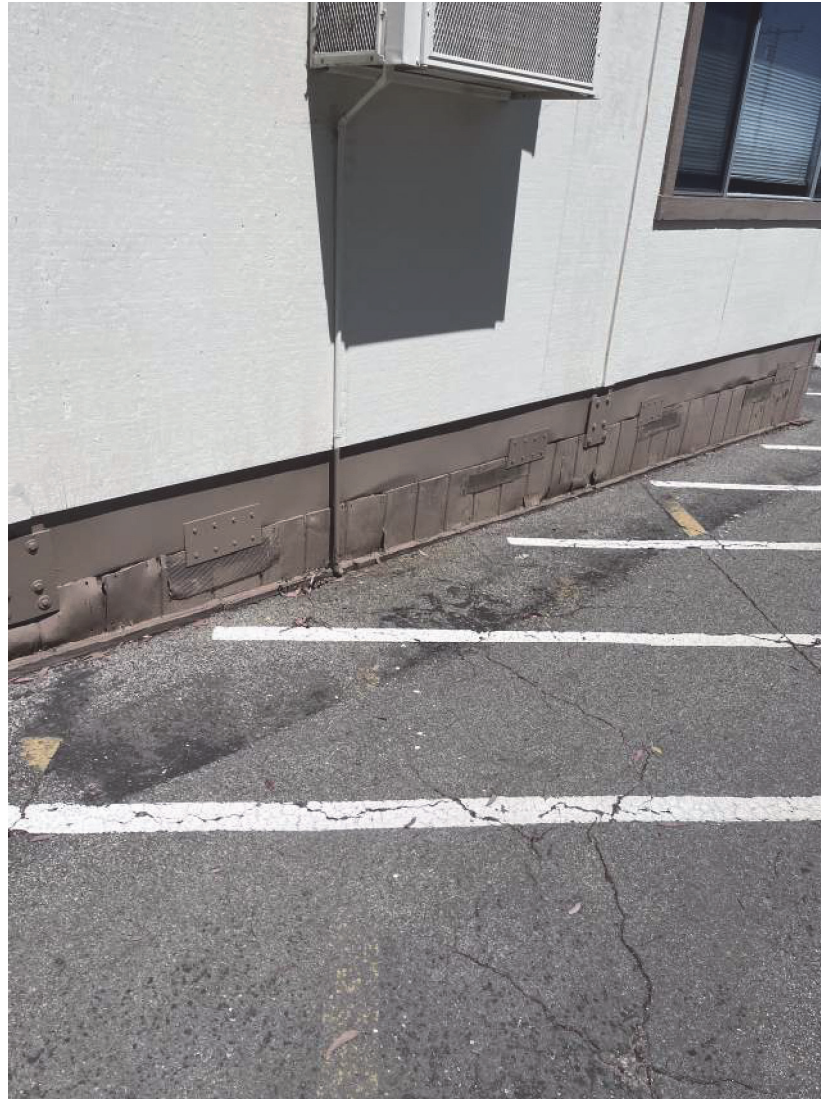
Slight Deterioration of Cripple Wall Sheathing
