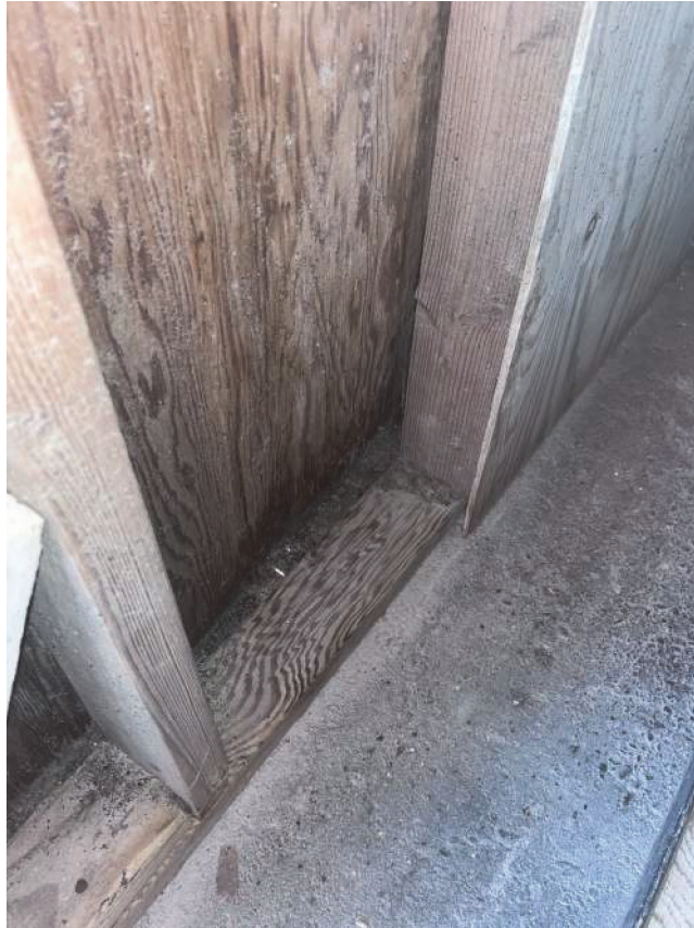
Building 37 - Damage to Sill Plate
