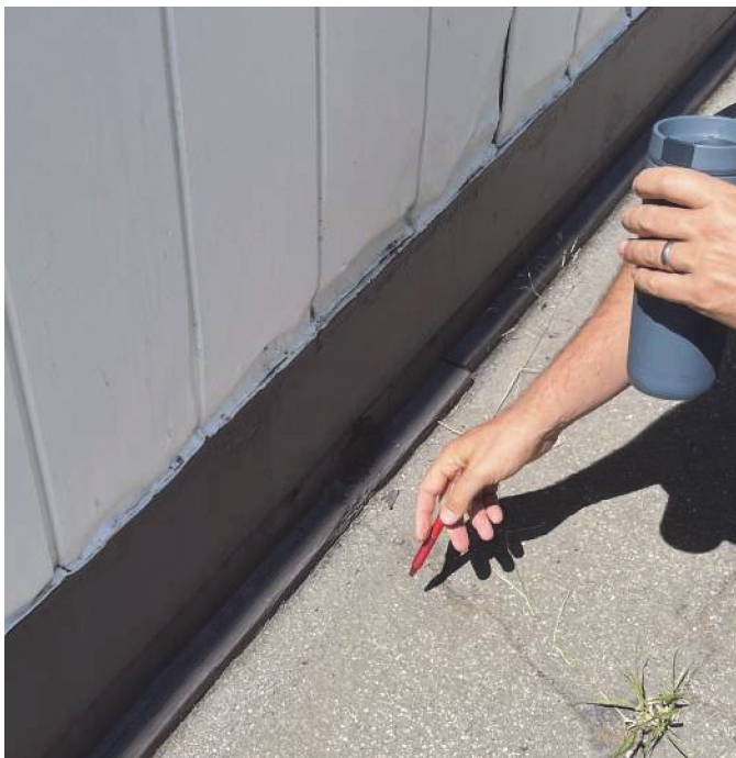
Damage to Plywood Skirting
