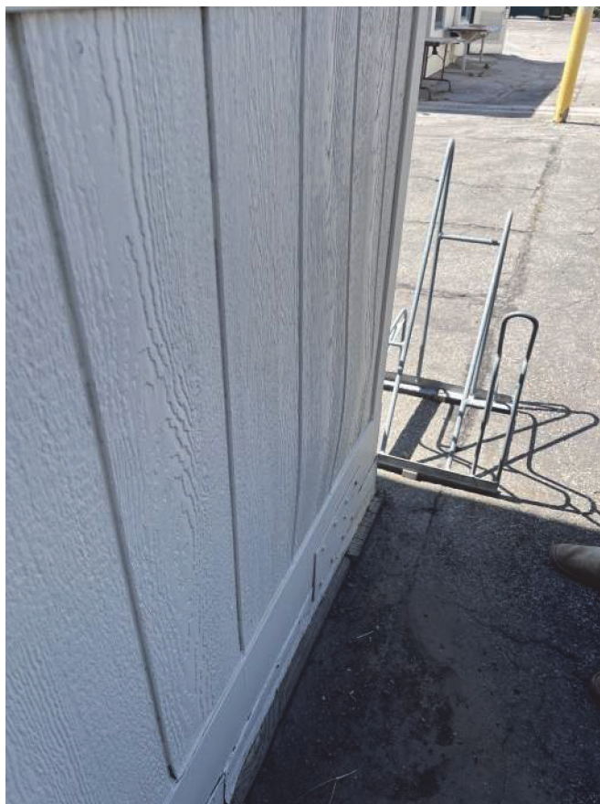
Damage to Metal Framing @ Foundation
