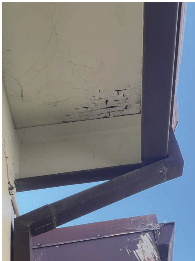
Damage to Plywood Roof Sheathing
