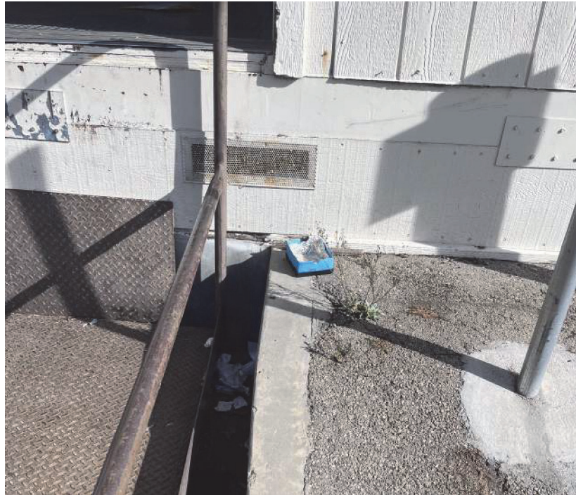
Deterioration of Wood Sill-On-Ground
