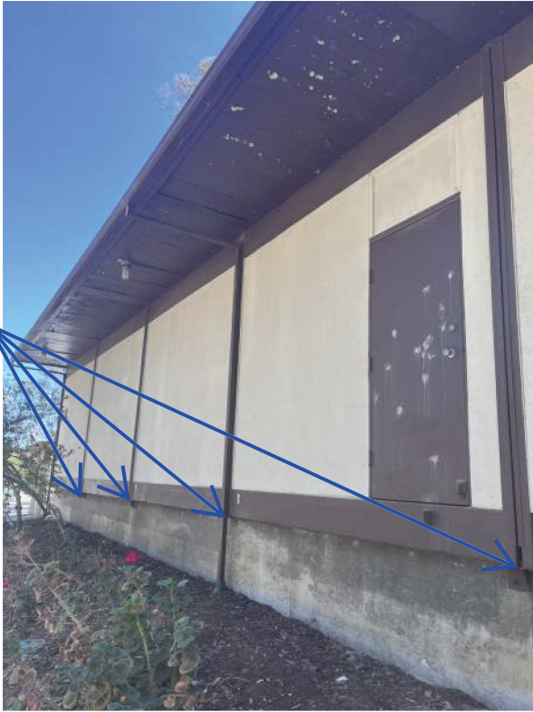
Inadequate Footing Anchorage
