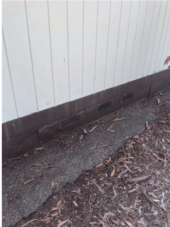
Slight Deterioration Cripple Wall Sheathing
