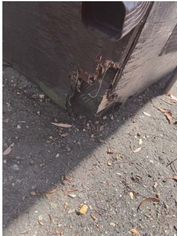
Slight Deterioration Cripple Wall Sheathing
