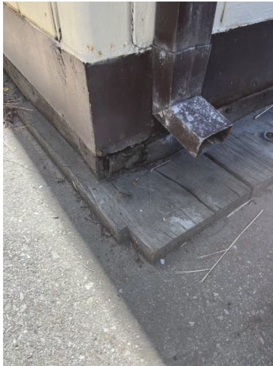
Damage to Plywood Skirting
